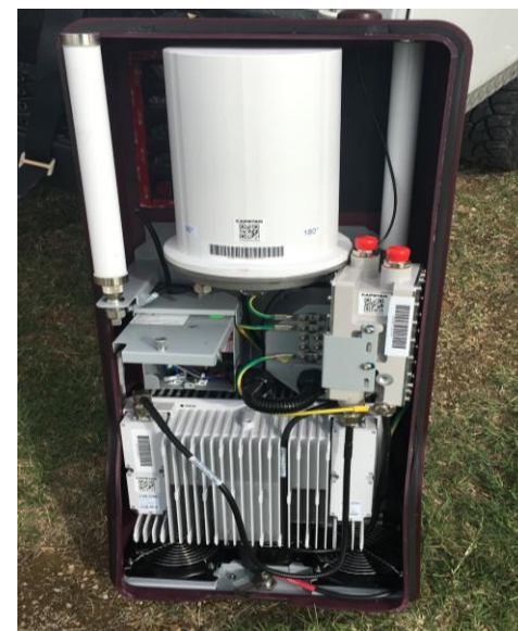
Inside of Cabinet
